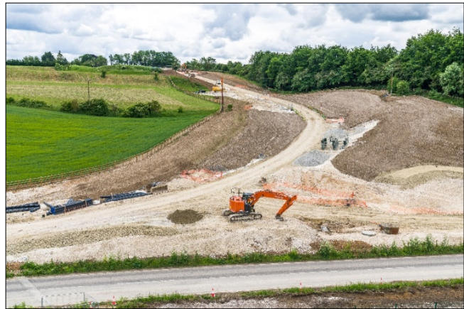
Progress on the Maidstone Road/Oad Street link taken from our site compound looking up.
