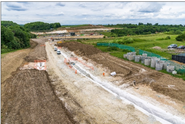
Progress on the Maidstone Road/Oad Street link taken from the top of the hill looking down towards the A249.
